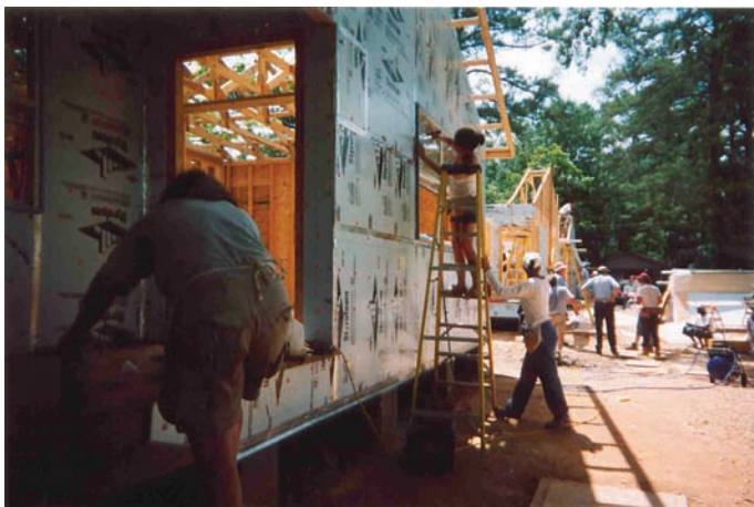
Pictured are volunteers building a Habitat for Humanity home in Covington, Louisiana.
